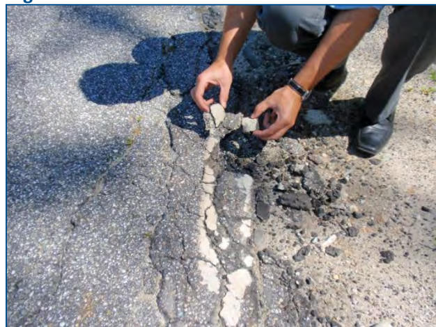
Figure 6.1: Poor Surface Condition – NH Route 127
