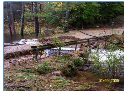
Figure 8.23: Canterbury Road Washout and Flooding, 2005
